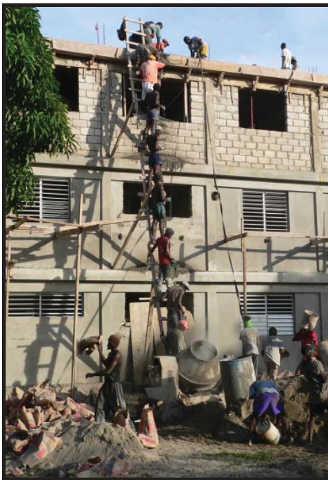
Workers build the 3rd story of the James Stine College with a concrete assembly line.
